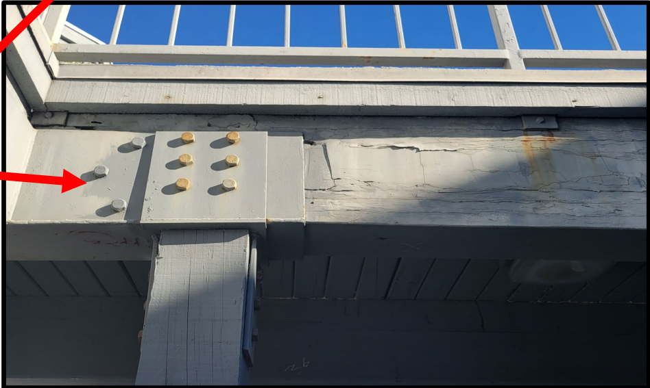
Old shoring and continued failure
