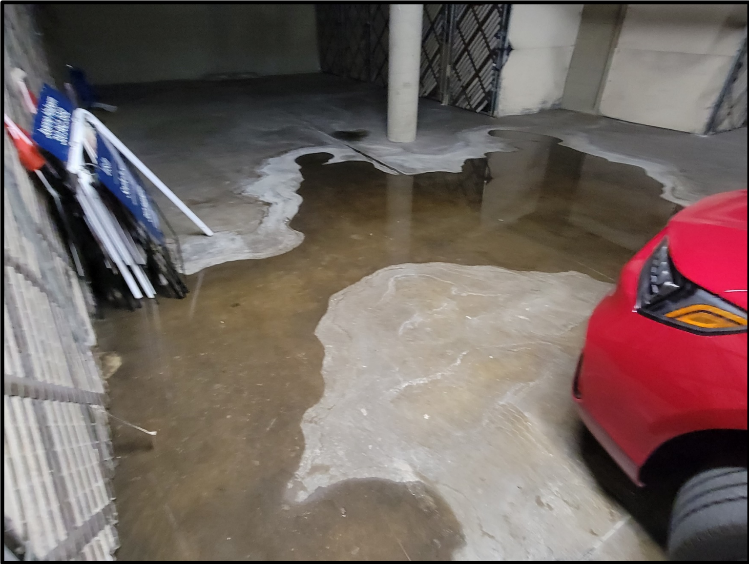
Water seeping in through garage walls.
